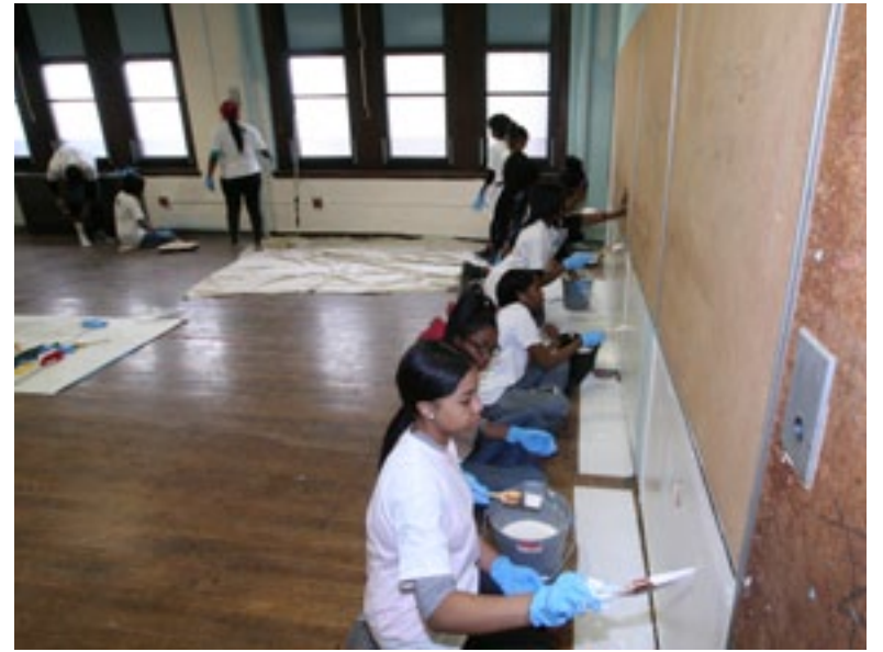
Students from Vaux Big Picture High School work on touching up the walls in one of the classrooms at the school to prepare for future expansions. 100 people volunteered for the event, including PHA residents, financial planners from the Fidato Group, recruiters from Penn State, and contracting partners TN Ward.
