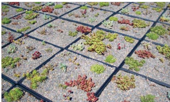
Tiny seedlings planted in the roofing at Nellie Reynolds Gardens will eventually form a three-inch deep environmentally friendly carpet.
