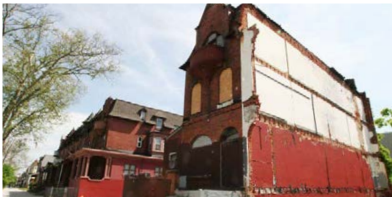
This dilapidated townhome at the corner of 33rd and Monument Streets is symbolic of the decay that has overtaken the historic Strawberry Mansion neighborhood. PHA's Strawberry Mansion-Oakdale development will renew the neighborhood and fill in the gaps on three blocks left after a number of decaying homes were demolished.
