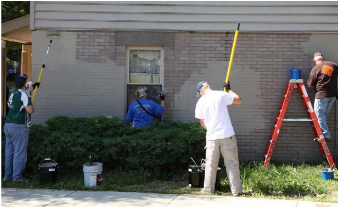
Volunteers from World Changers, a faith-based group that promotes community service, did painting, landscaping and other maintenance work at Raymond Rosen (shown here) and three other PHA sites. The group donated over $100,000 in labor during a four day visit to Philadelphia.
