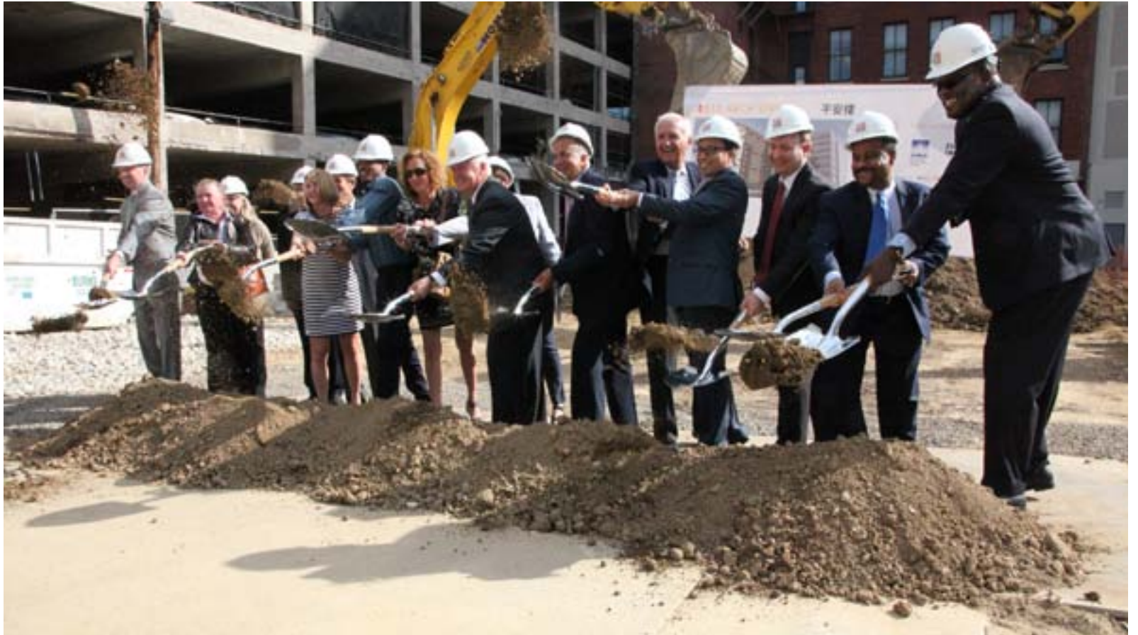
PHA President and CEO Kelvin Jeremiah (far right) joins Governor Tom Corbett and other state and local leaders at the groundbreaking for Project HOME's new development at 810 Arch Street in Chinatown. PHA has committed 50 Project-Based Vouchers to the development.
